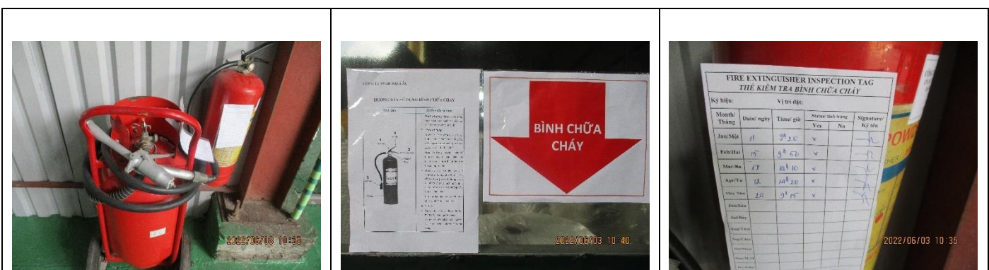
Fire Extinguishers #2 Visible Sign for Fire Extinguisher The Internal Inspection Records of the Fire Extinguisher
